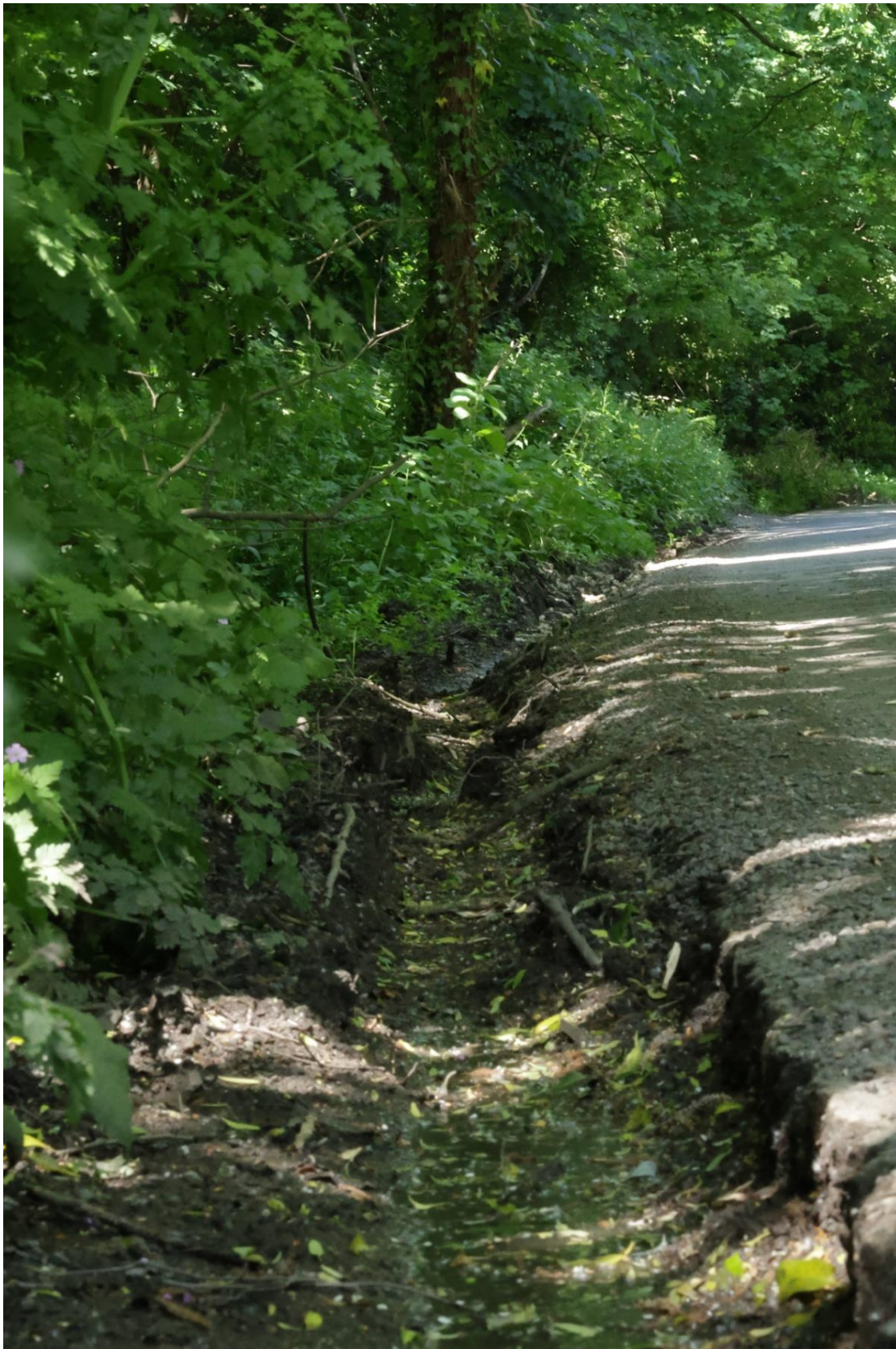
Figure A1.14 Erosion of verge on Rockbourne Road (May 2024)
