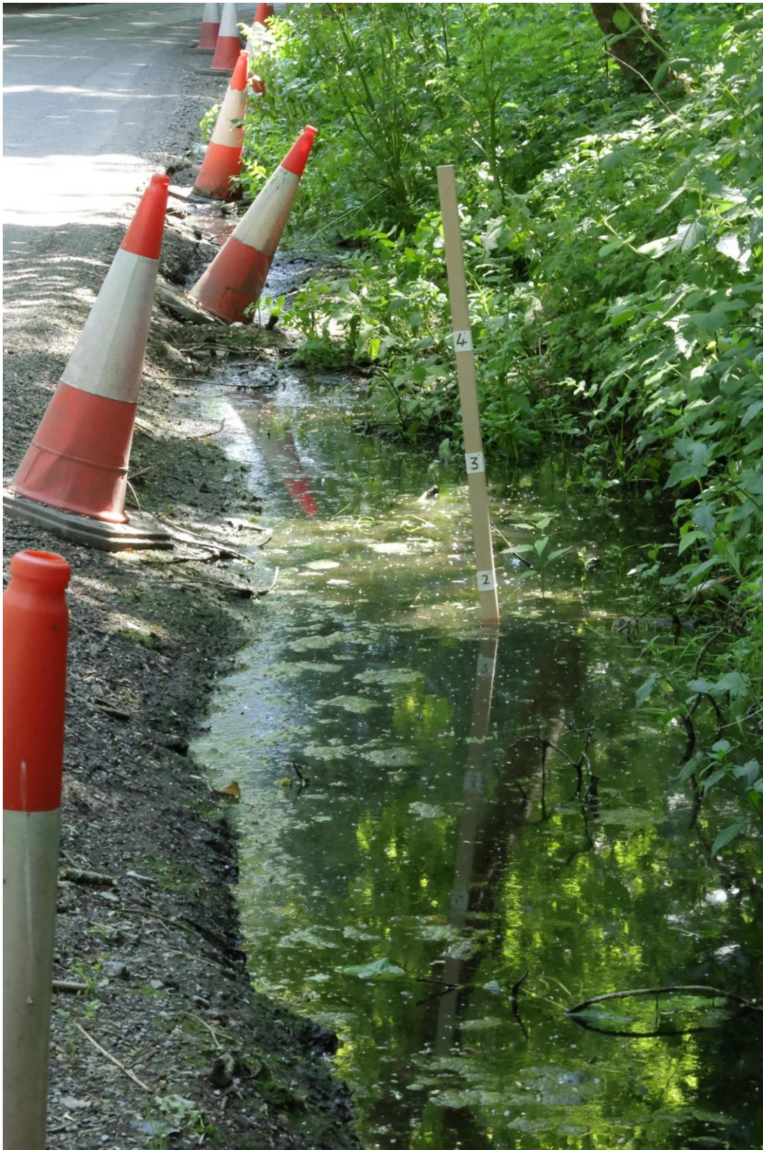
Figure A1.13 Erosion of verge on Rockbourne Road showing depth of about 3 feet (May 2024)
