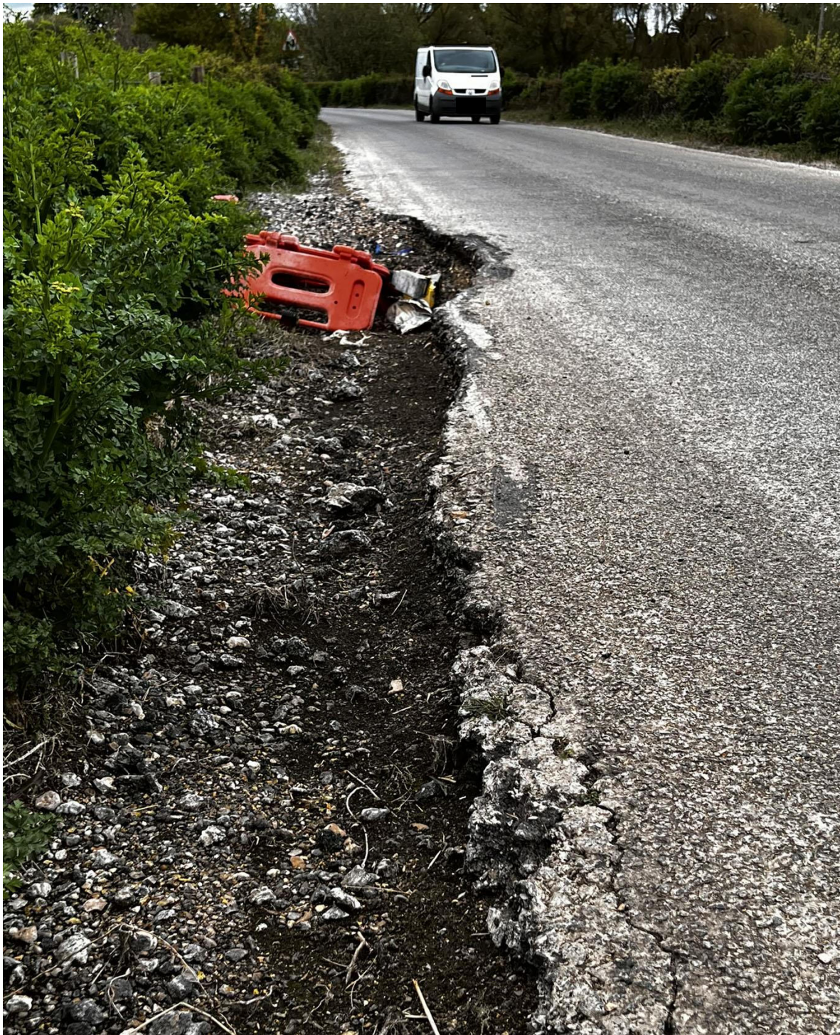
Figure A1.12: Erosion of pavement on Kent Lane (May 2024)
