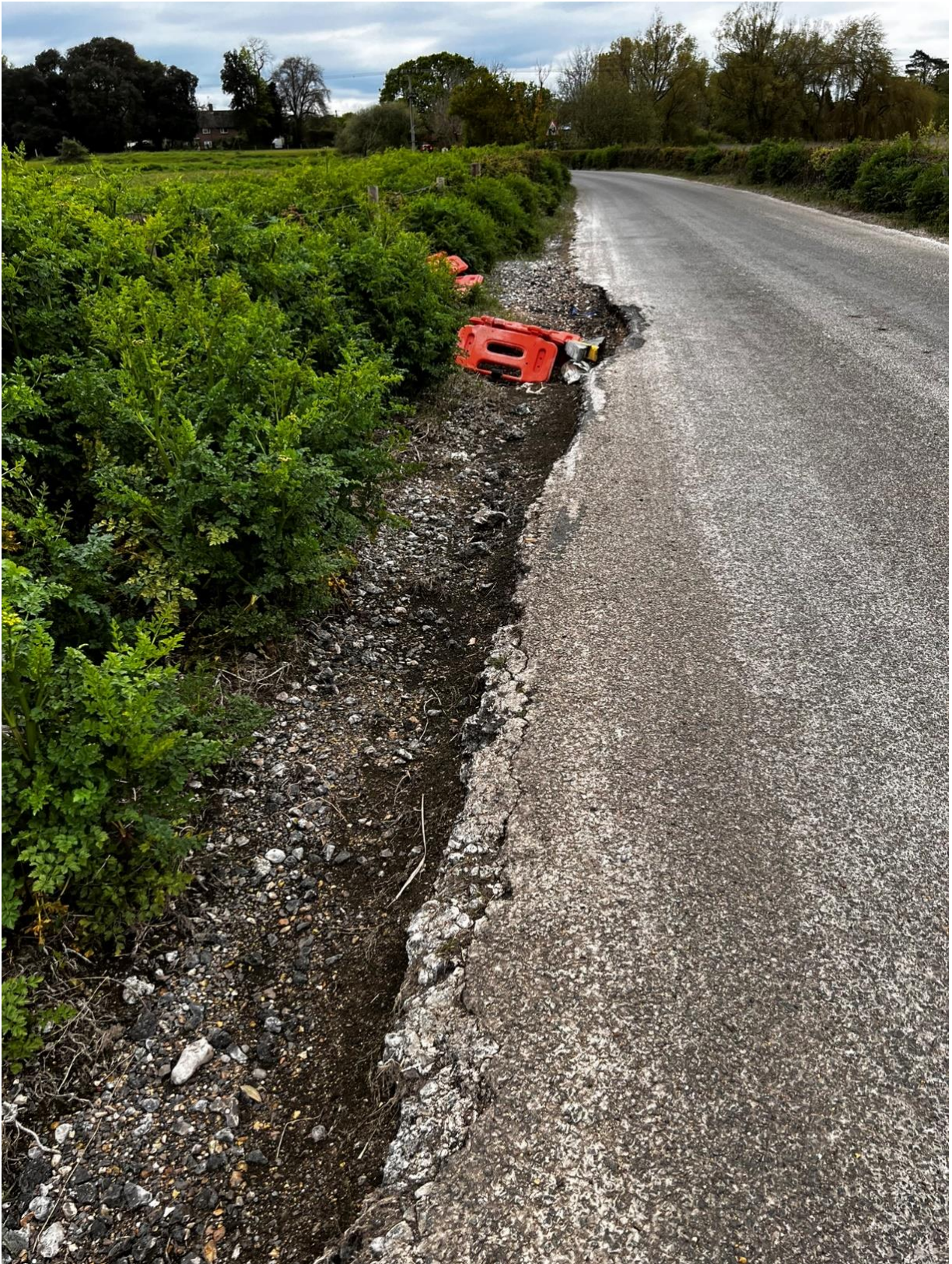
Figure A1.11: Erosion of pavement on Kent Lane (May 2024)
