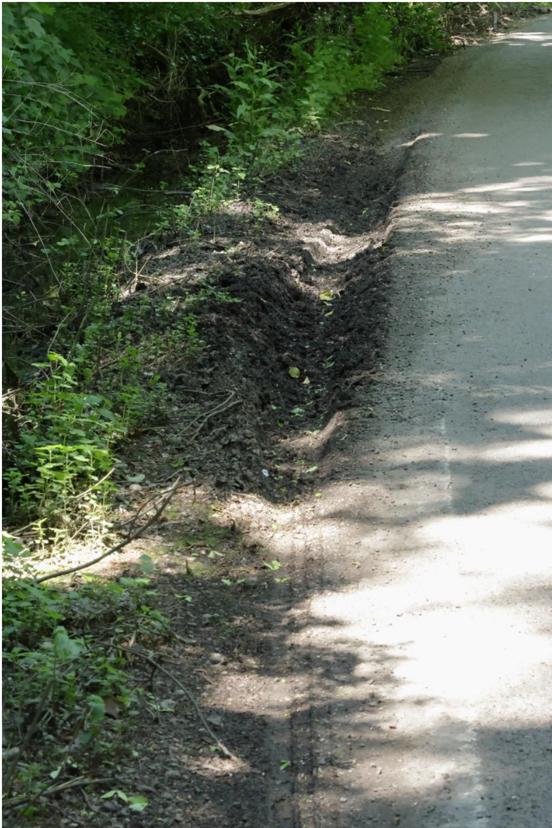
Figure A1.15 Erosion of verge on Rockbourne Road showing car tracks (May 2024)
